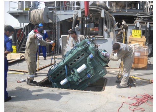
One of three diesel generators providing shipboard electrical service on USNS Catawba.
